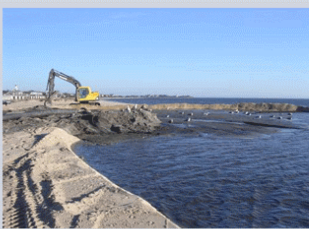
Dewatering basin designed for physical separation of sand and fine-grained dredge sediments at Craigville Beach, Barnstable, MA.
